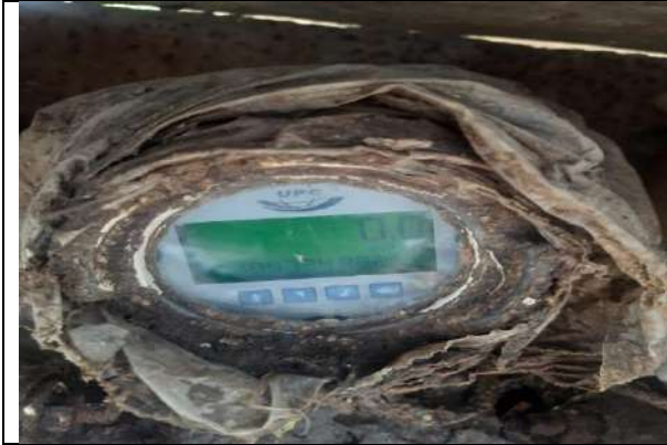
Flow meter installed at Borewell-1
