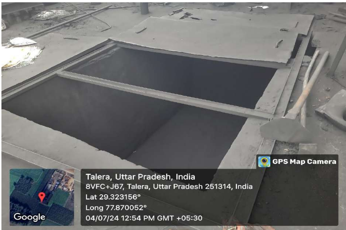
Figure 8 Char storage tank
