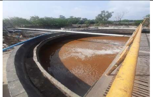
Treated effluent before recycling to process
