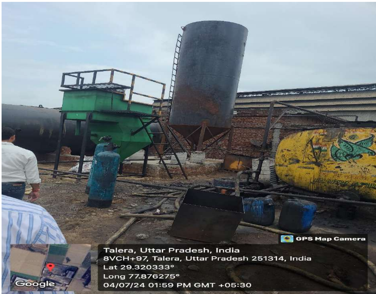
Figure 3 ETP system yet to be installed
