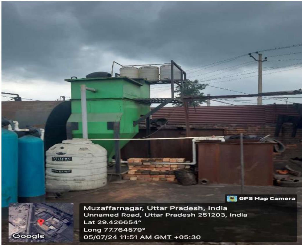
Figure 7 Installed ETP under trial
