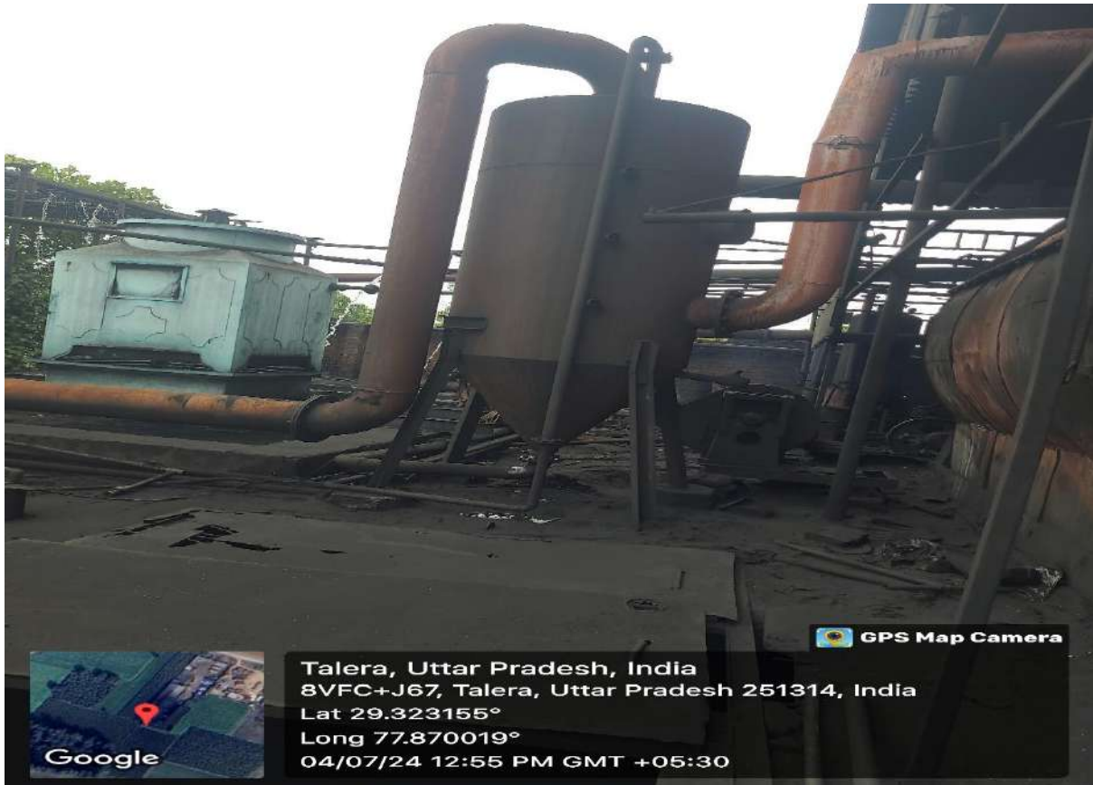
Figure 7 Wet scrubber found leaking at the time of inspection
