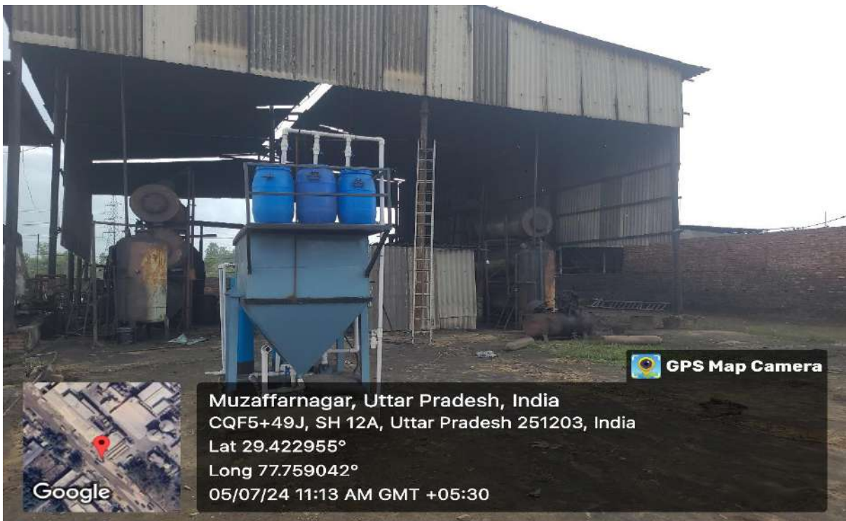
Figure 6 ETP under commissioning
