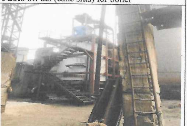
Photo 10: Gasifier for plastic waste
