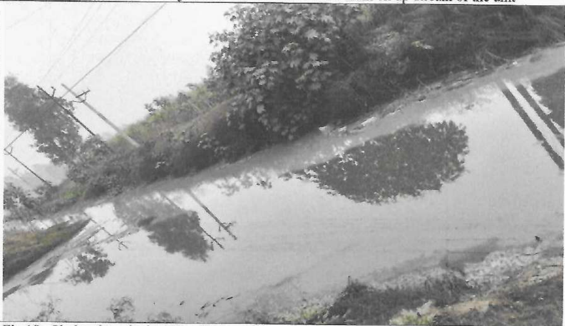
Fig.18: Sludge deposits in Dhandhera drain on down-stream side
