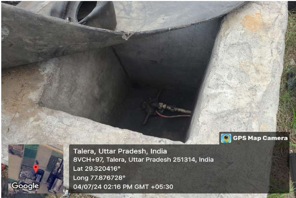
Figure 10 Borewell inside unit's premises
