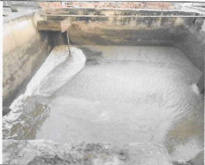
Photo 3: ETP inlet channel
