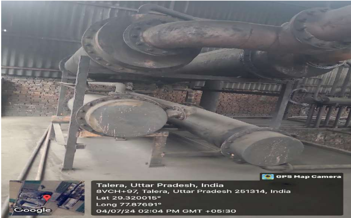
Figure 8 Oil and gas compressor system
