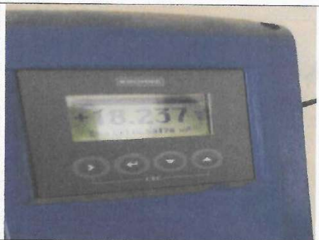
Photo 2: Borewell - flow meter
