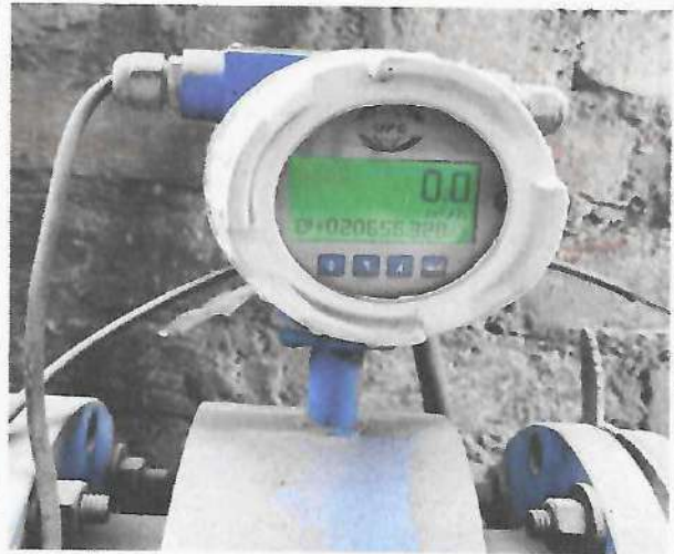
Flowmeter reading of Borewell No. 2
