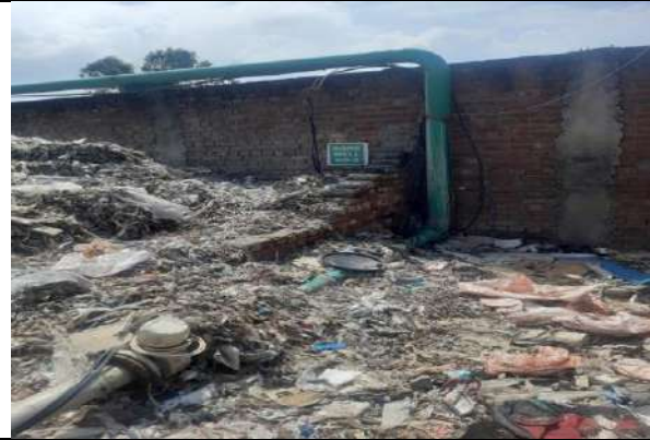
Borewell-2 defunct flow meter
