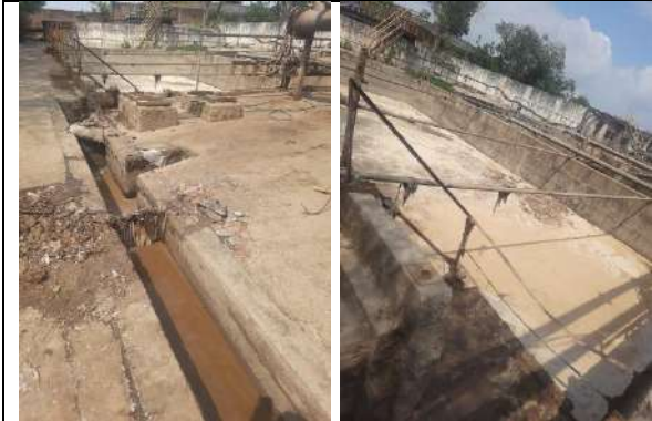
ETP Inlet & Equalization tank
