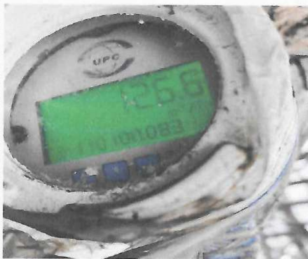
Flowmeter reading of ETP inlet
